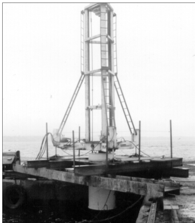
Figure 2 Test apparatus consisting of 0.6 MN Statnamic device, hydraulic catching mechanism, platform, and underwater reaction mass assembly (shown above water).
