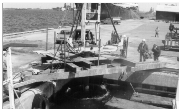
Figure 3 View of test setup clearly showing the support platform spanning the corner of the dock.
